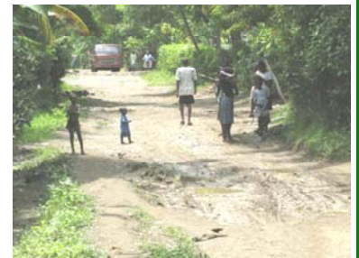
Detour on main road between Port-au-Prince and Cap-Hatien. Many roads in Haiti are now being rebuilt, but even where cement exists, numerous giant potholes limit top speeds to 30-40 mph.
